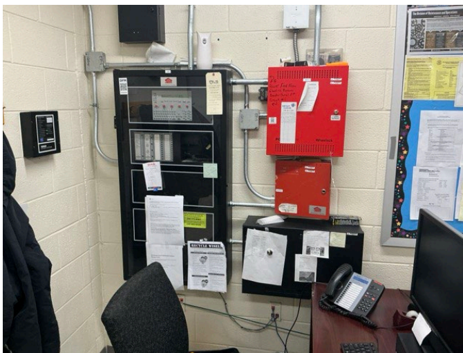
33 - FIRE ALARM PANEL
