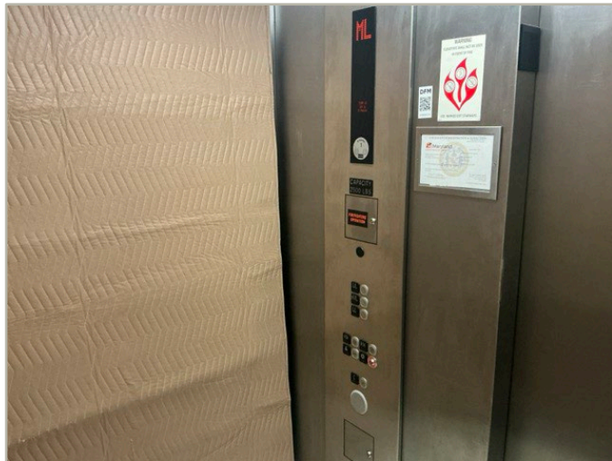
IN-CAB CONTROLS/EMERGENCY CALL PANEL
