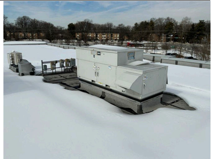
26 - PACKAGED ROOFTOP UNIT
