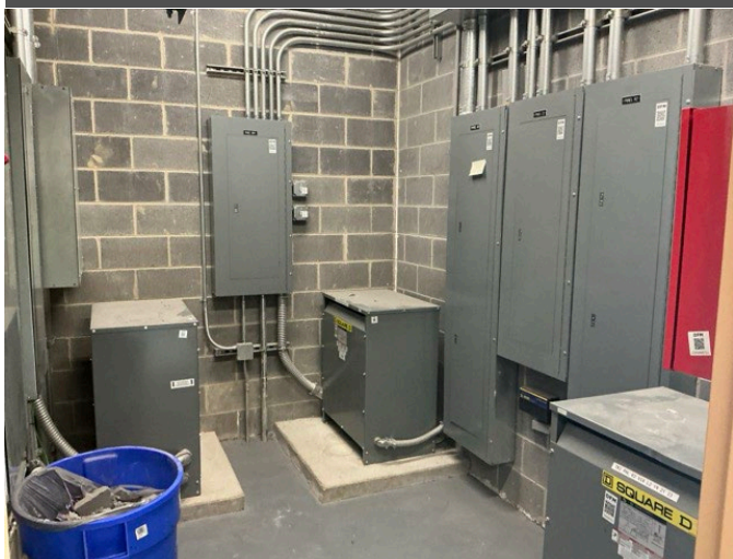
31 - SECONDARY ELECTRICAL ROOM
