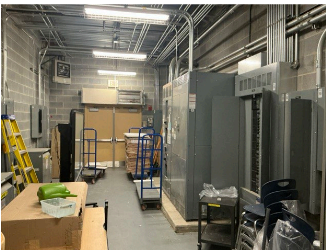
29 - MAIN ELECTRICAL ROOM
